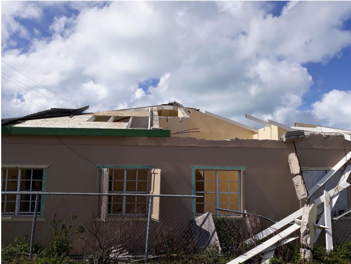
Barbuda Codrington Fire station – Showing all 4 modes of roof failure from hurricane winds. 1. Metal sheet separation from the ply roof deck. 2 Ply roof deck separation from the rafters. 3. Rafters breaking off with sections of roof deck & sheet. 4 Rafters torn out of the walls and pulling out masonry in the process. Note the horizontal reinforcing bar laid in the concrete top of the masonry wall failed in sections - due to a lack of vertical strapping.
