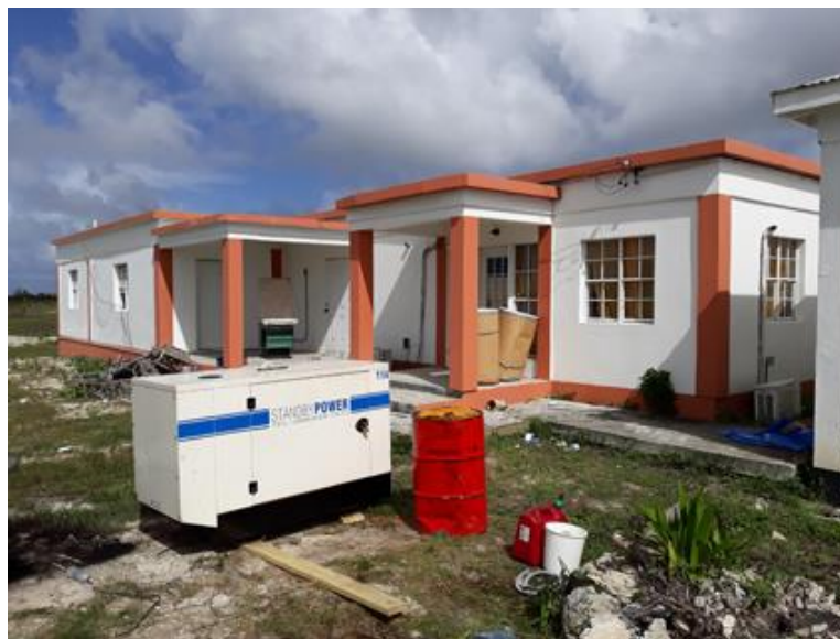
Codrington Hospital – Parts of the hospital had flat concrete roofs, which were not affected by the hurricane
