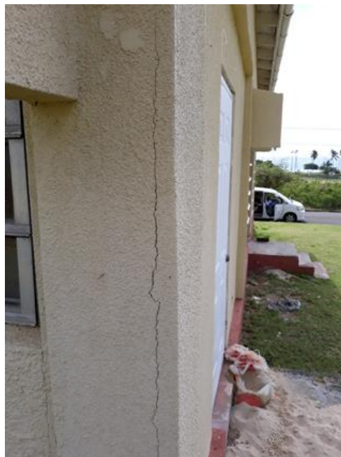
Old Road – Cracked concrete column, probably due to reinforcing steel corrosion
