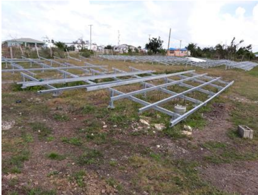
Codrington Power station 100kWp solar array – The hurricane destroyed 95% of the ground mounted panels
