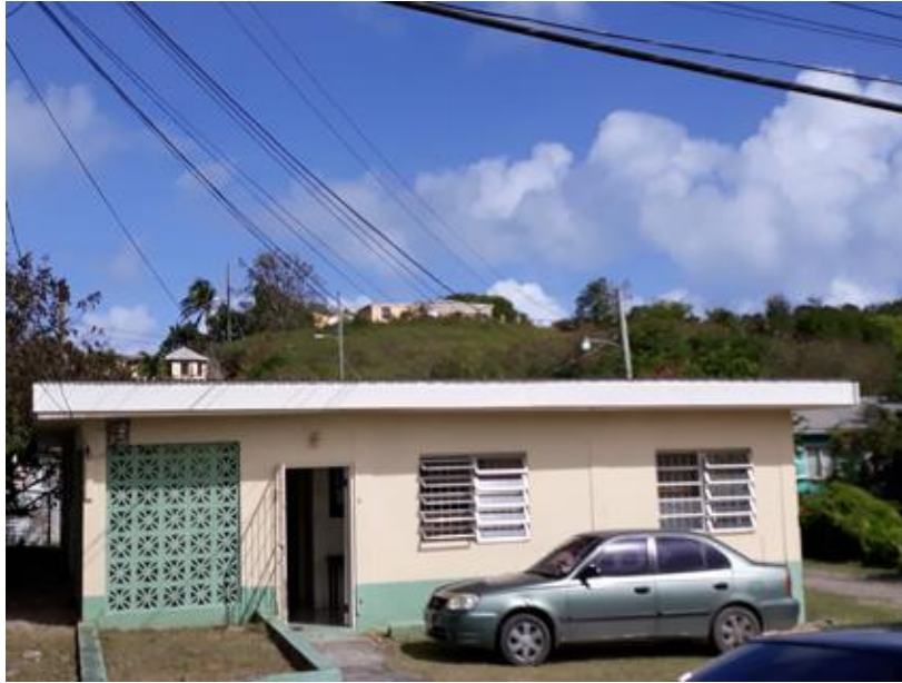
Parham clinic – showing obstructing powerlines
