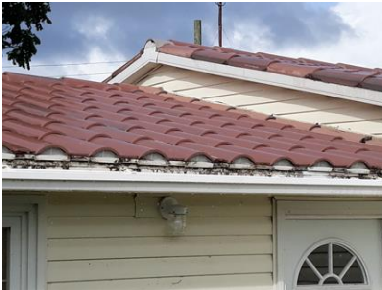
Good Shepherd home for children – A plastic roof on a plastic clad structure: the structure is fully concealed and visible only through partial dismantling.
