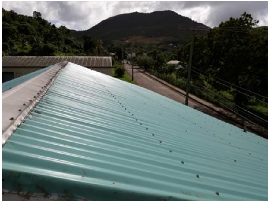
Bendalls clinic – A recently replaced metal roof with roof screws, fixed into battens or traverse rafters and only limited fixings into the pitched rafters. Roof integrity is controlled by the rafters.
