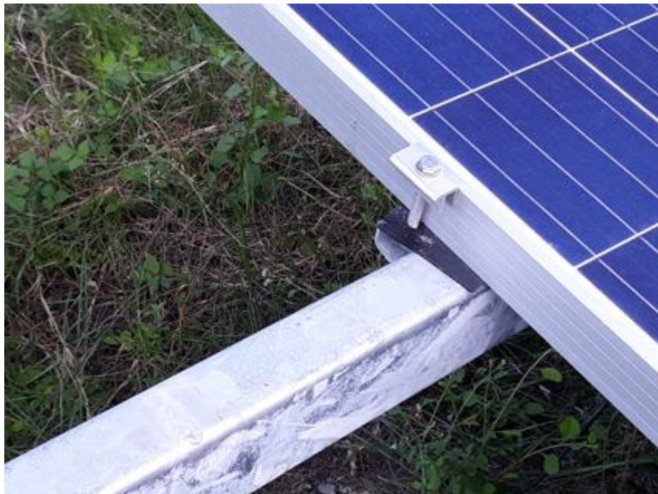
Codrington array – The alloy fixings between the PV panels and the racks can be the weakest point for wind vulnerability
