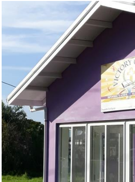
Victory Centre – Recent build showing traverse rafters, ply deck and extended eaves
