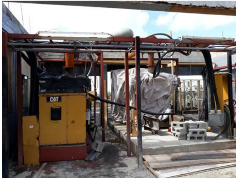
Codrington power station – The generator house was deroofed. Critical infrastructure such as this should be strongly hardened against hurricane winds
