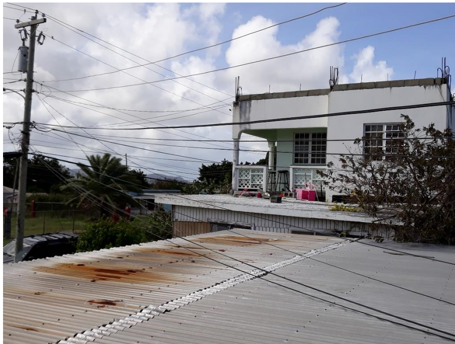
Powerlines lying on the roof of Parhams clinic
