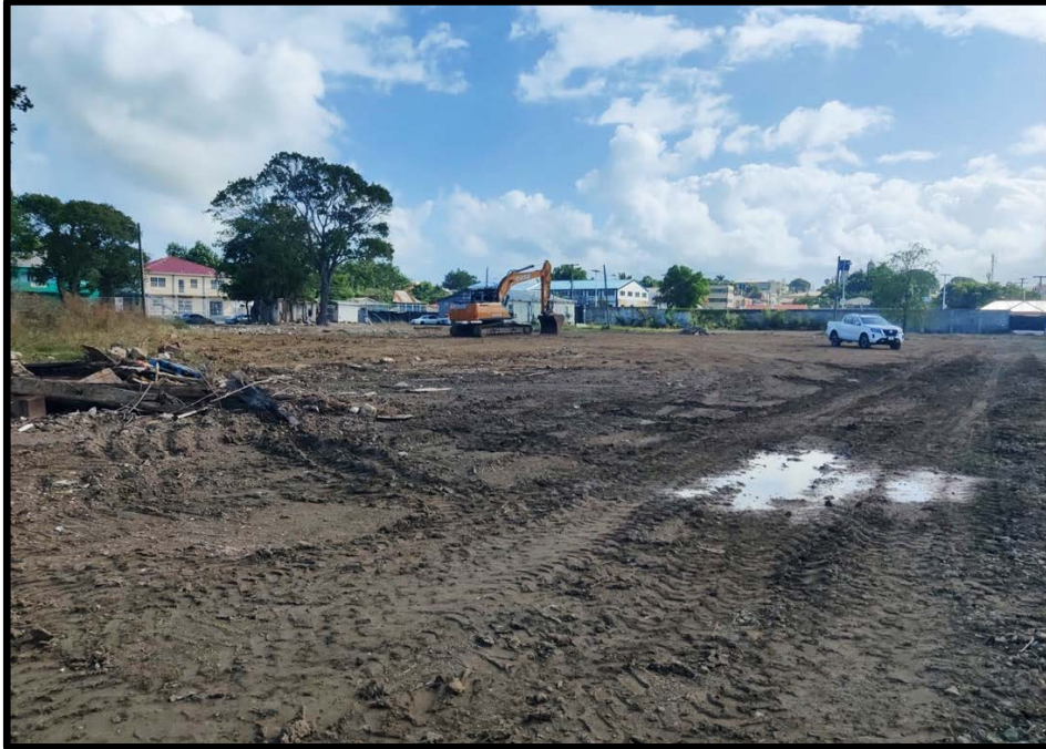
Figure 7: Overview of General Site Conditions including evidence of ponding
