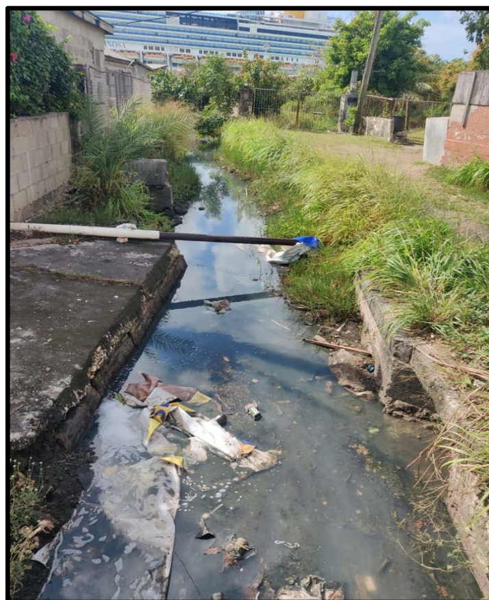
Figure 9: Open Community drain from north of project site and west of Barnes Funeral Home
