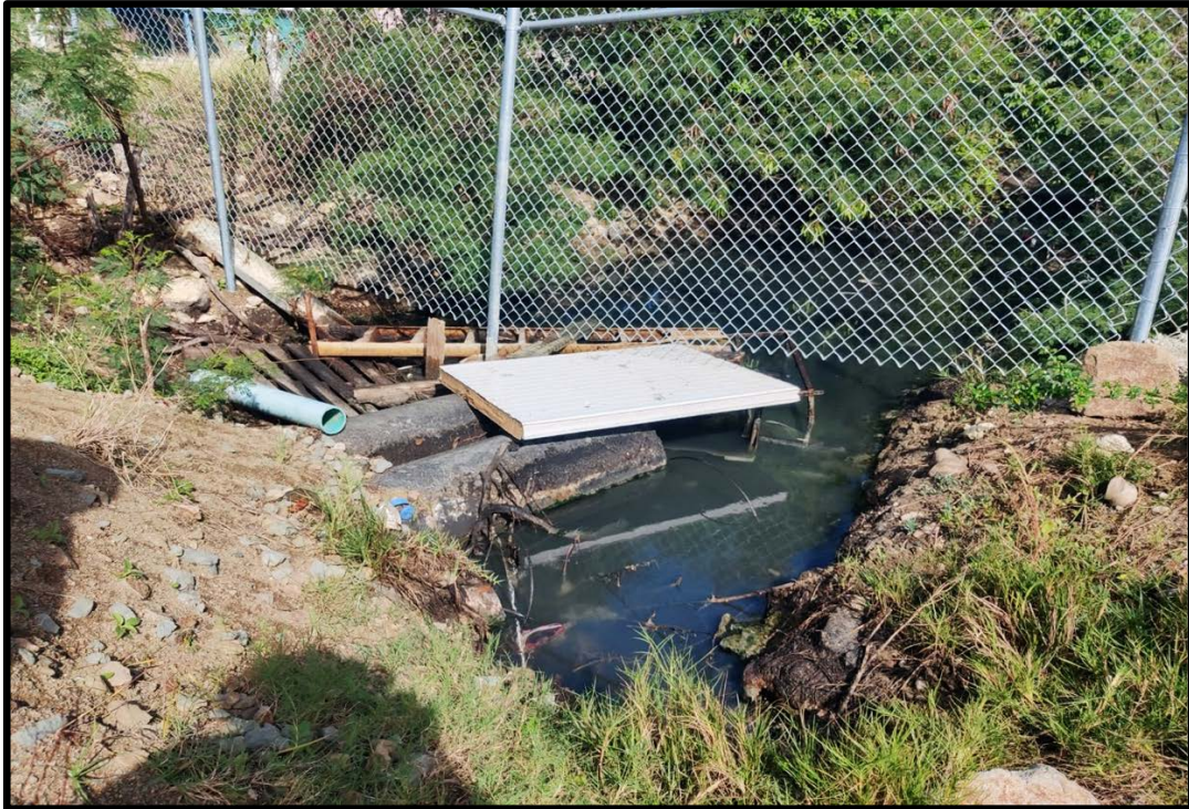
Figure 10: Observed drainage pipes within project site suggesting direction flow into community drain
